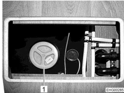
Fig. 118 Cleaning opening (waste water tank)
