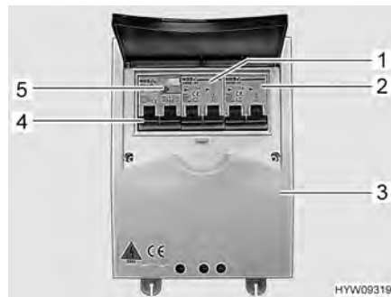
Fig. 65 Safety cut-out and FI-switch (240 V fuse box)
