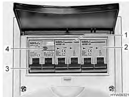
Fig. 69 Safety cut-out and FI-switch (240 V fuse box)
